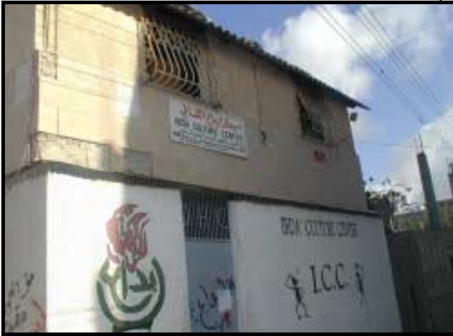
PHOTO: Ibdaa building totally burned from inside; computer-lab, library, office and stores destroyed
